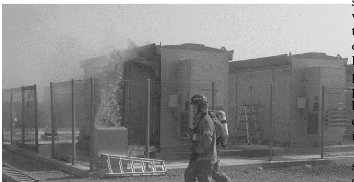
Fig. 8 Battery energy storage system on fire [11]
